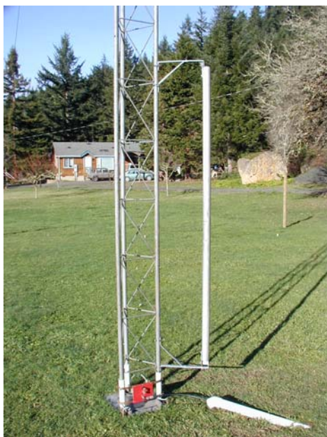
Figure 7, example of a shunt loop at the base of a tower. The loop is resonated with a series capacitor to form a parallel resonant trap, decoupling the base and the tower over a narrow range of frequencies.
