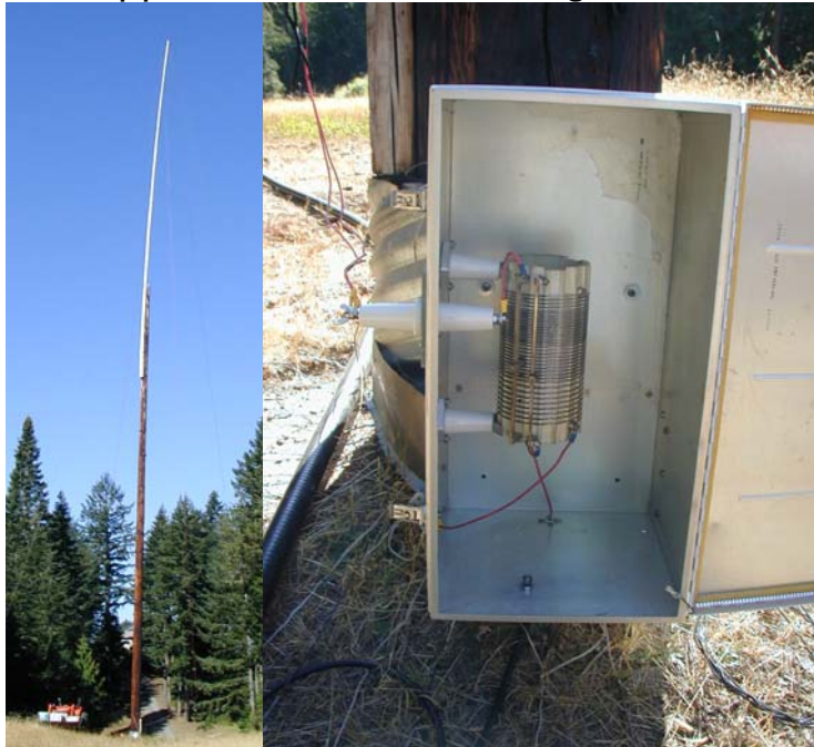
Figure 2, WD2XSH/20 600m antenna support and base tuning inductor.
